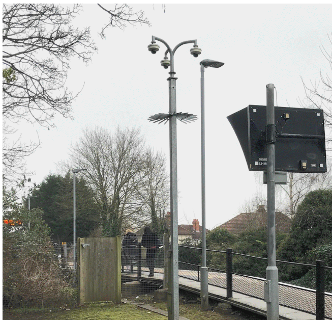
CCTV mast at Furze Platt
